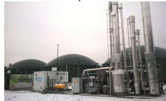
Digesters, upgrading unit and compressor unit
